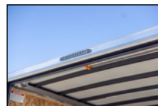
Bowed Roof Crossmembers
