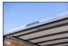
Bowed Roof Crossmembers
